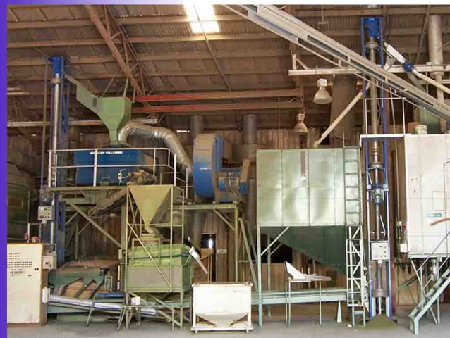
Two 6" (150mm) Olds Elevators conveying beans into various downstream processes.
